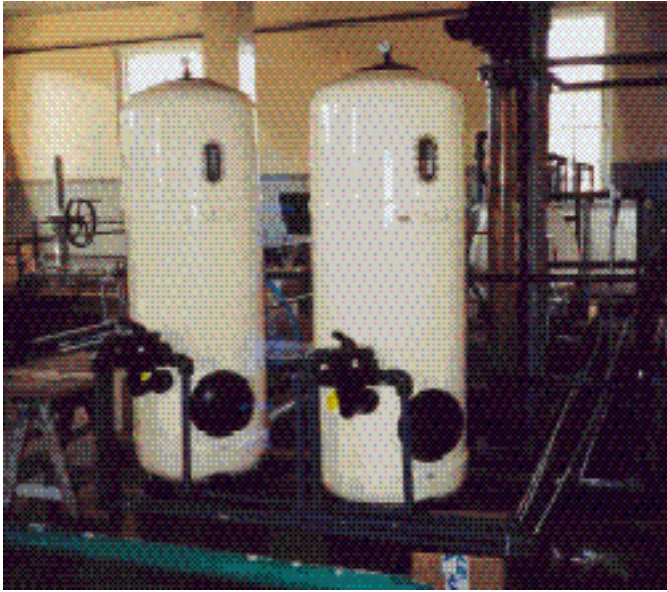
Figure 2.2 AFM and Sand Filter Test Bed Columns - Site K
