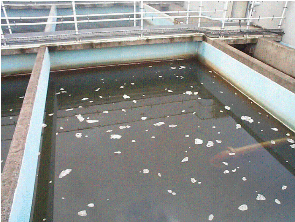
Rapid gravity filter for drinking water treatment
